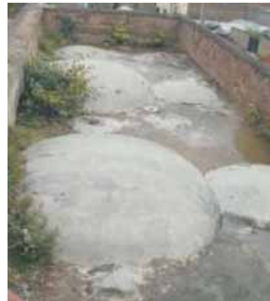
Roofs of buildings in need of maintenance
