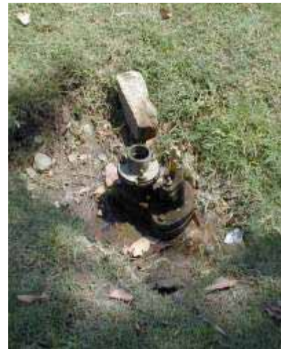
Poorly maintained valves for watering the gardens
