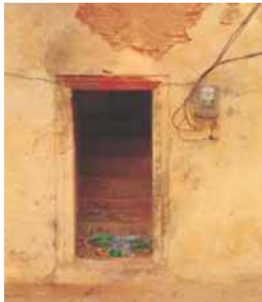
Deteriorating fabric and evidence of poor maintenance
